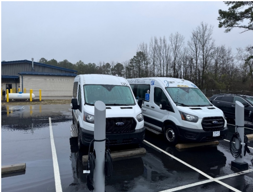
Figure 17. Existing electrical level 2 chargers
